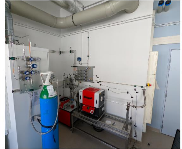
Furnace & gaz handling system
