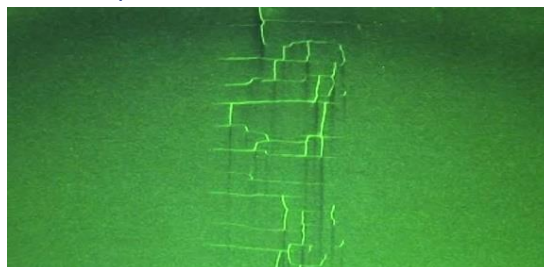
Magnetic particles UV image of surface breaking cracks
